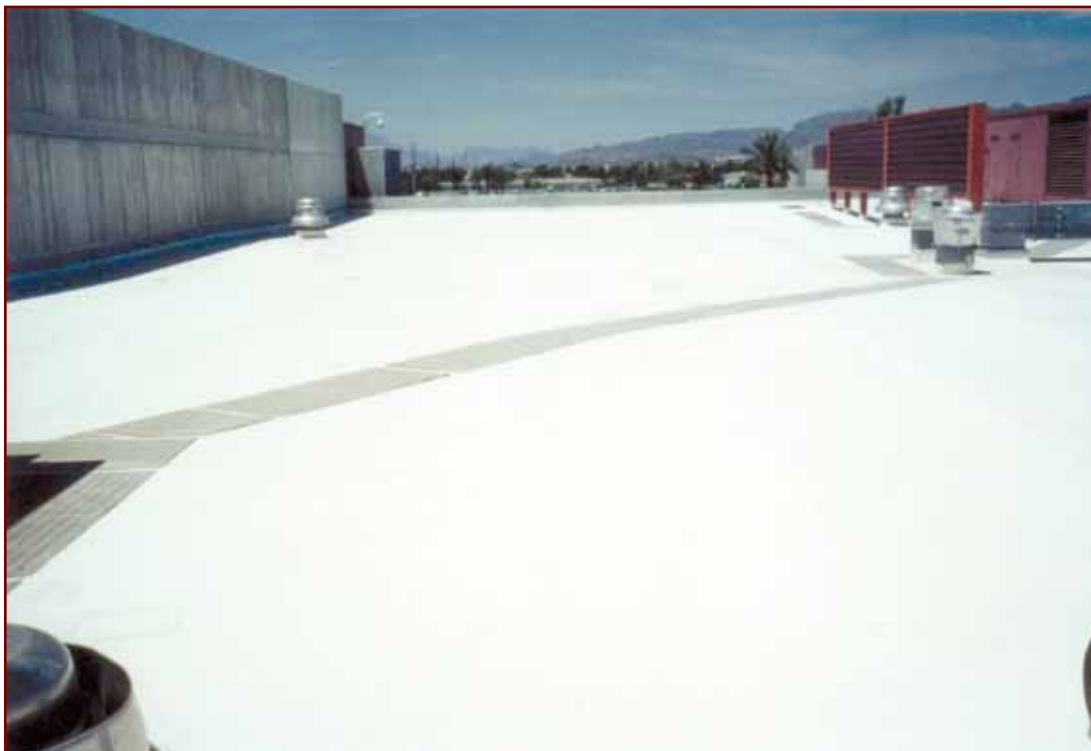
The granulated modified bitumen roof on this Intel facility in Chandler, Arizona, was coated with an elastomeric white coating.
